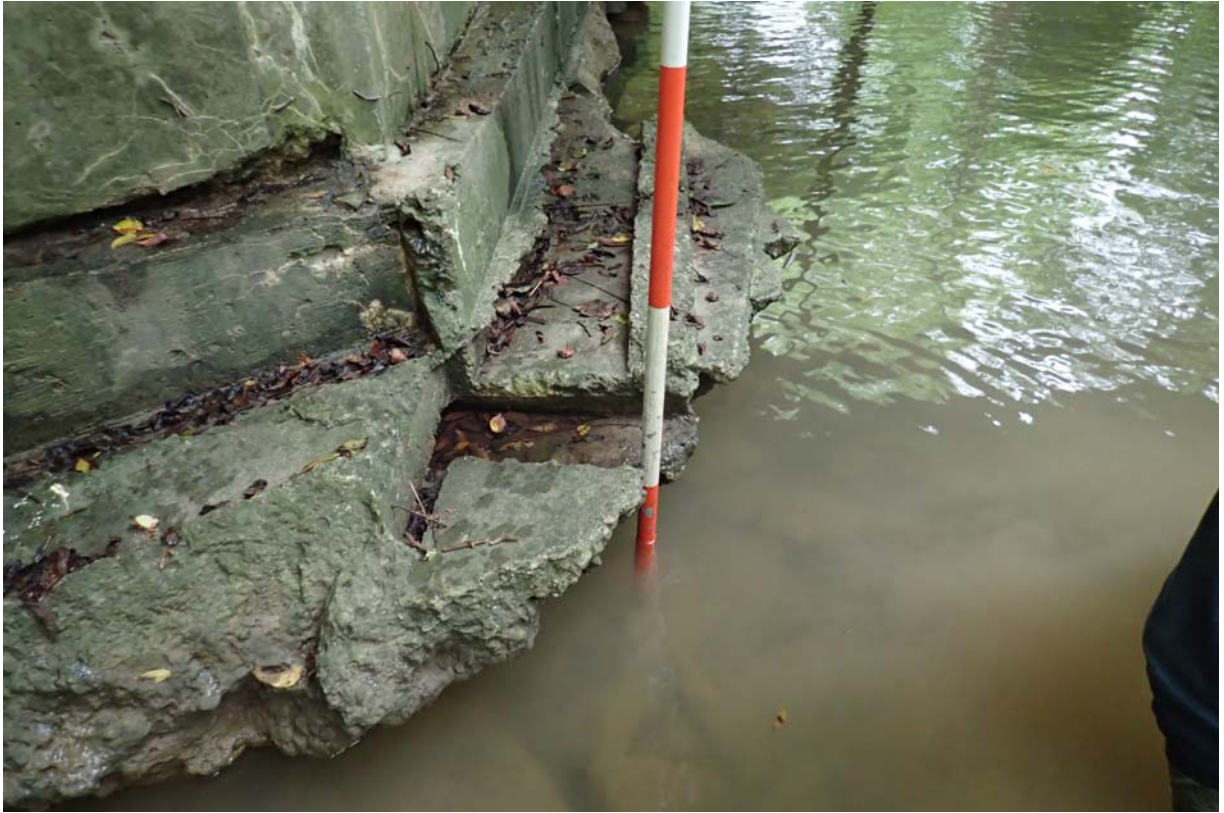
Up to 12" of vertical undermining at the upstream end of the west abutments footing/apron.
