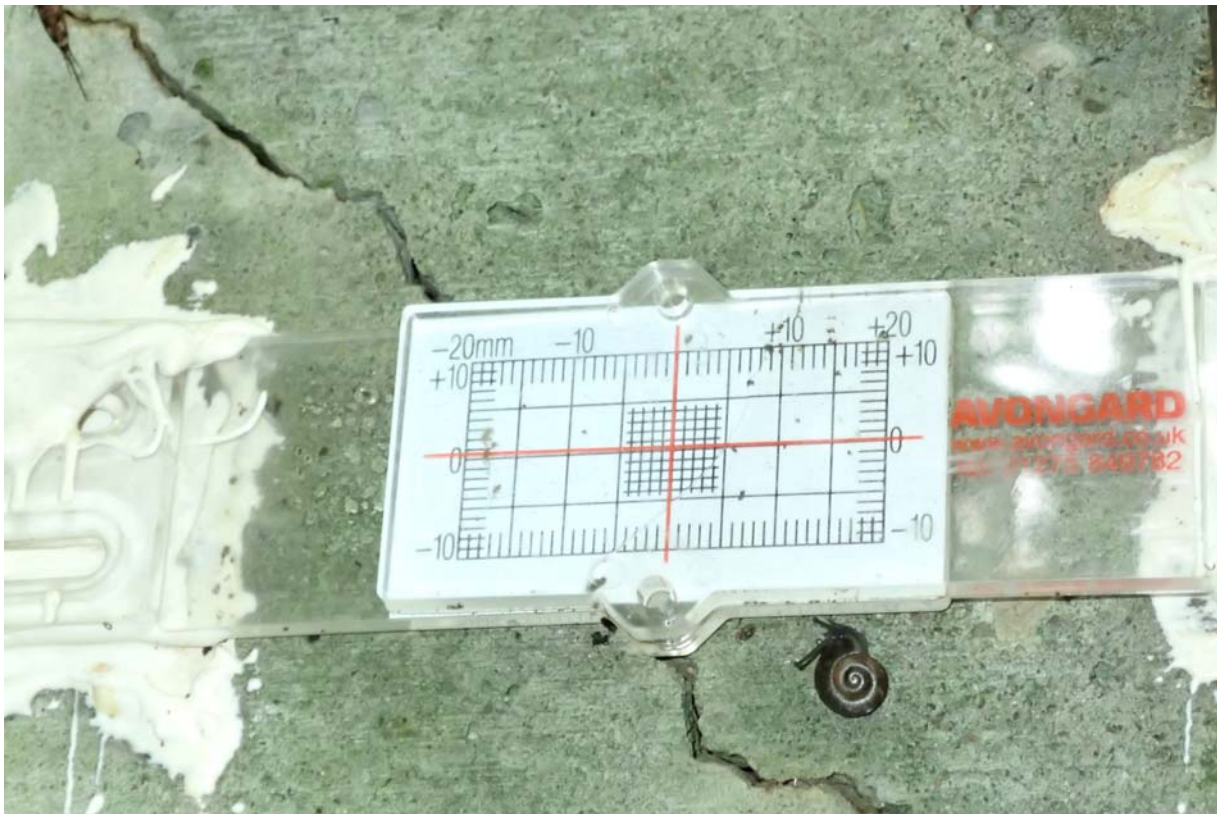
View of the crack gauge on the forward crack (toward stream) in the upstream west wingwall.
