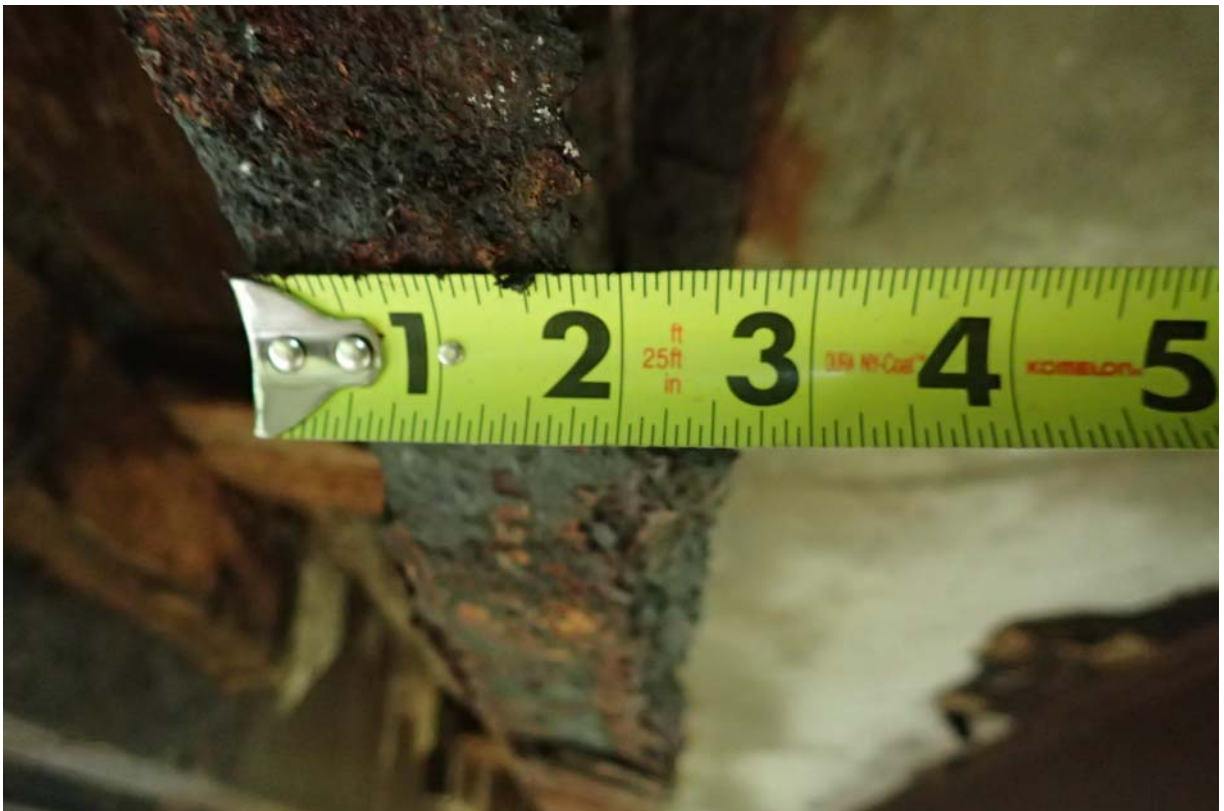
Heavy section loss within the width and thickness of beam 4s bottom flange ~ 7' from the west abutment.
