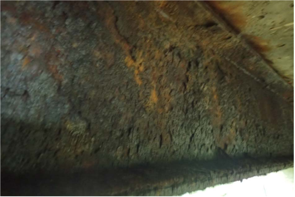
Heavy corrosion of beam 6 from upstream near the west abutment.
