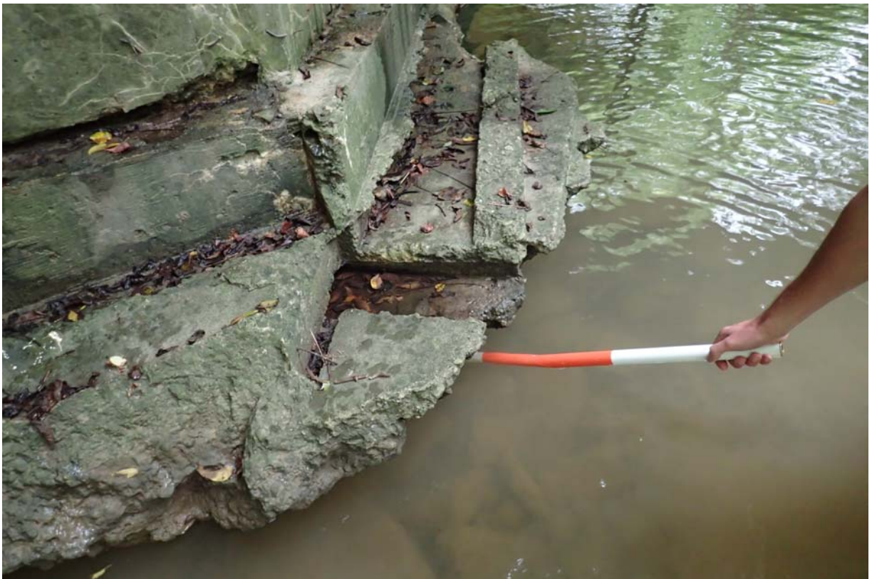
Up to 24" of horizontal undermining at the upstream end of the west abutments footing/apron.
