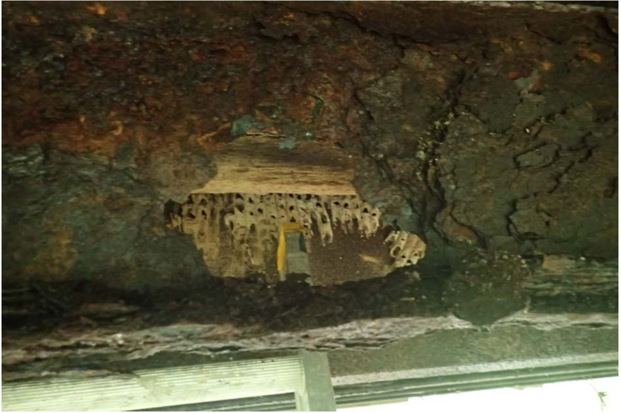
Large rust through hole in the web of beam 4 from upstream ~ 7' from the west abutment.
