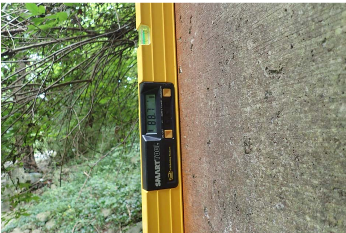
Smart level measurement at the downstream end of the east abutment.
