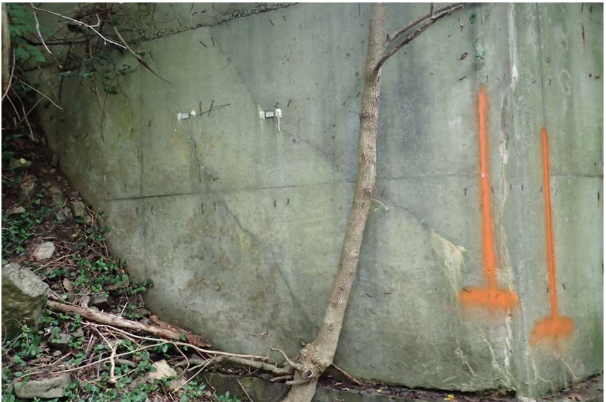
Moderate sized (1/16" typical) diagonal cracking in the upstream west wingwall.
