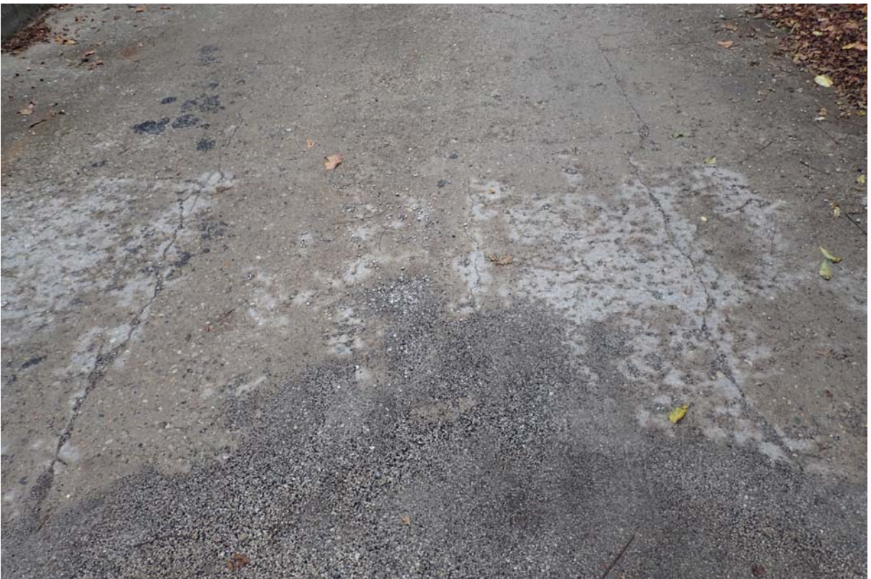
Moderate longitudinal cracking at the west end of the deck.
