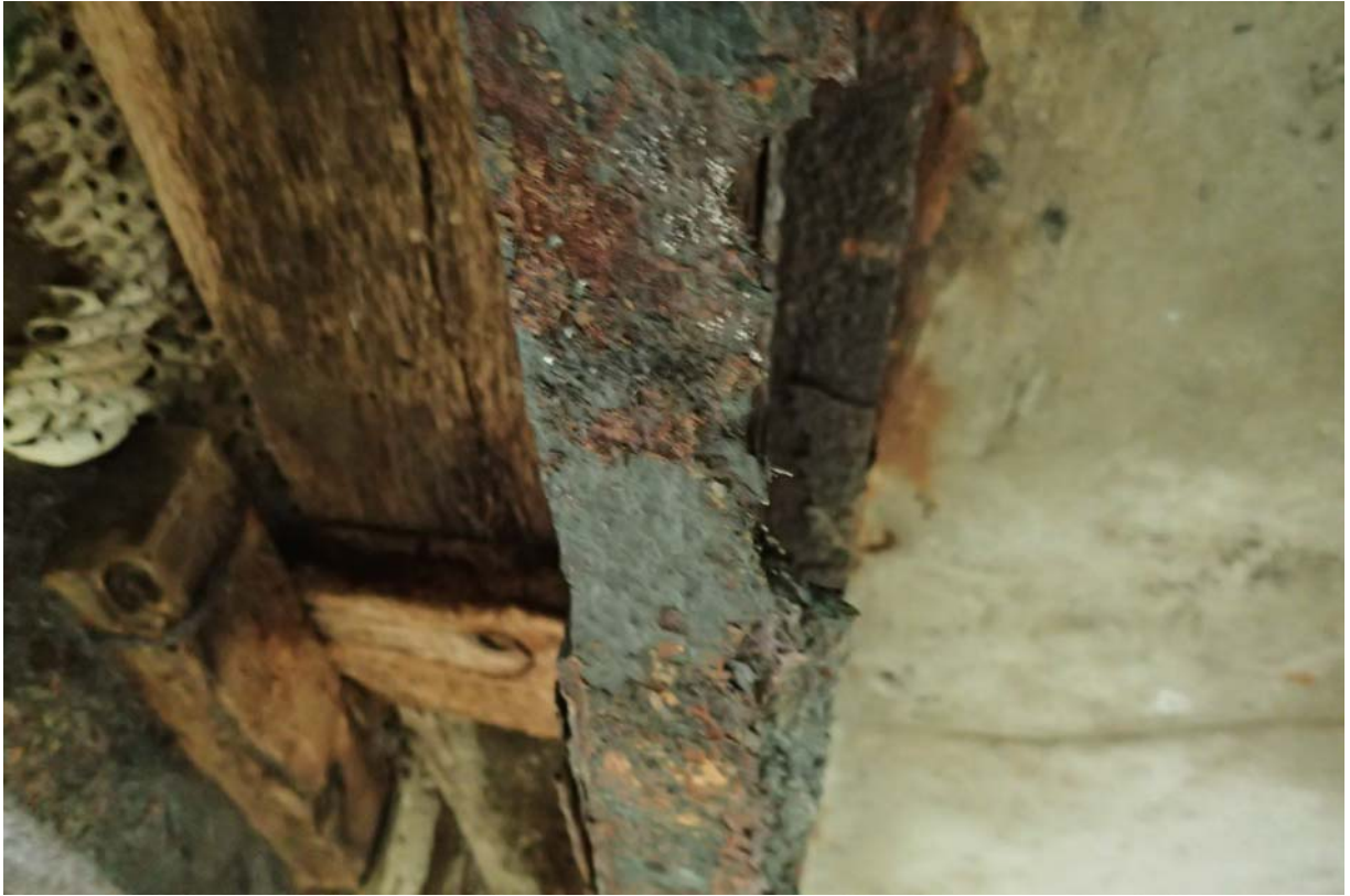
Heavy section loss within the width and thickness of beam 4s bottom flange ~ 7' from the west abutment.
