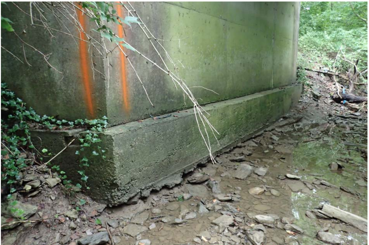
Minor undermining (horizontally up to 5") along the downstream 1/2 of the east abutments footing.
