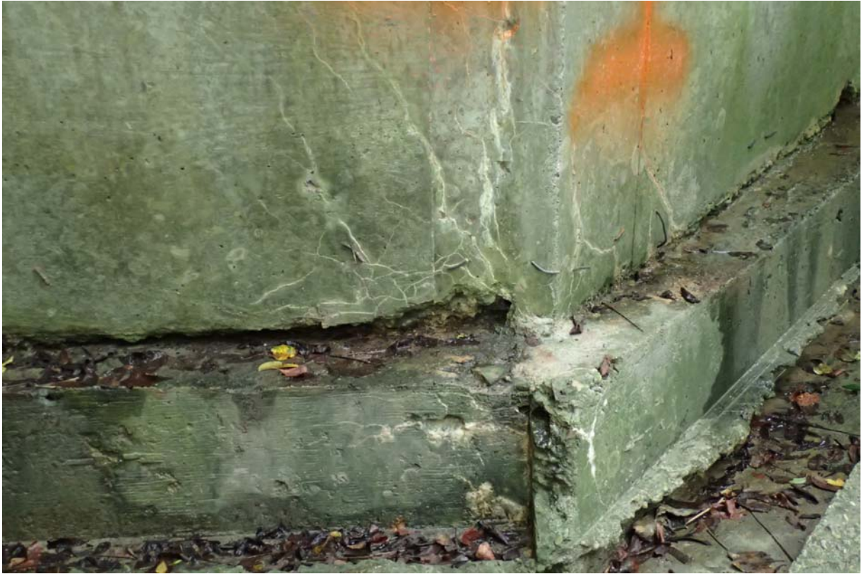
Moderate to heavy intensity of minor sized cracking and moderate spalling at the upstream west abutment/wingwall interface.
