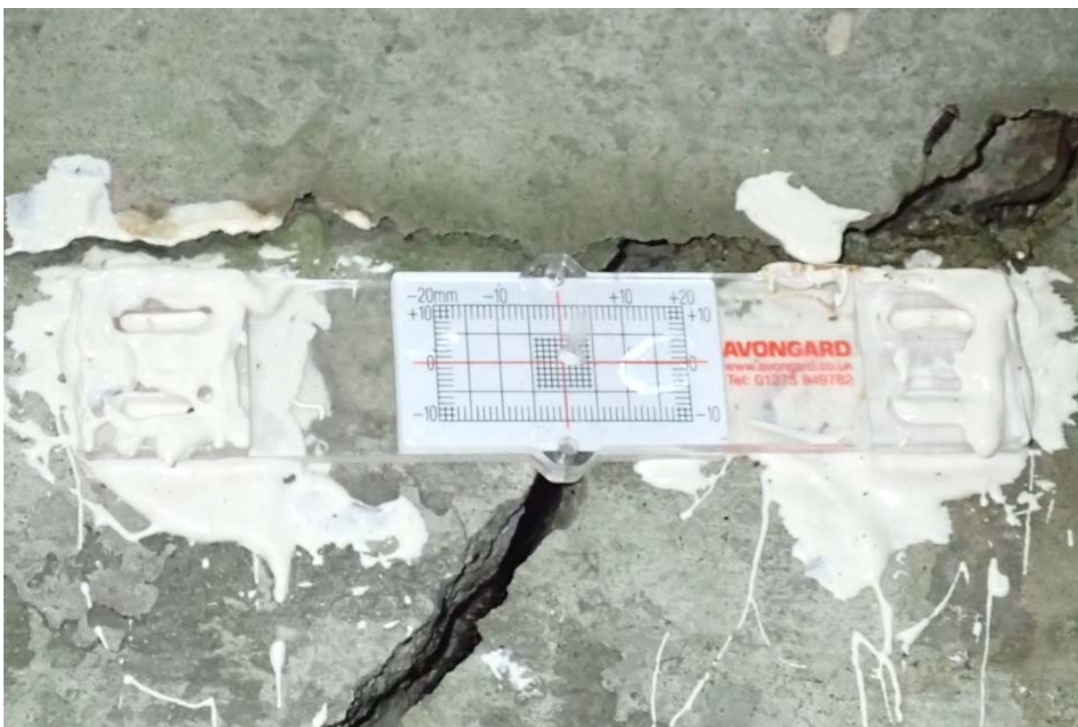
Crack gauge monitoring moderate diagonal cracking ( \sim 3/16'' - 1/4'' ) in the downstream west wingwall.
