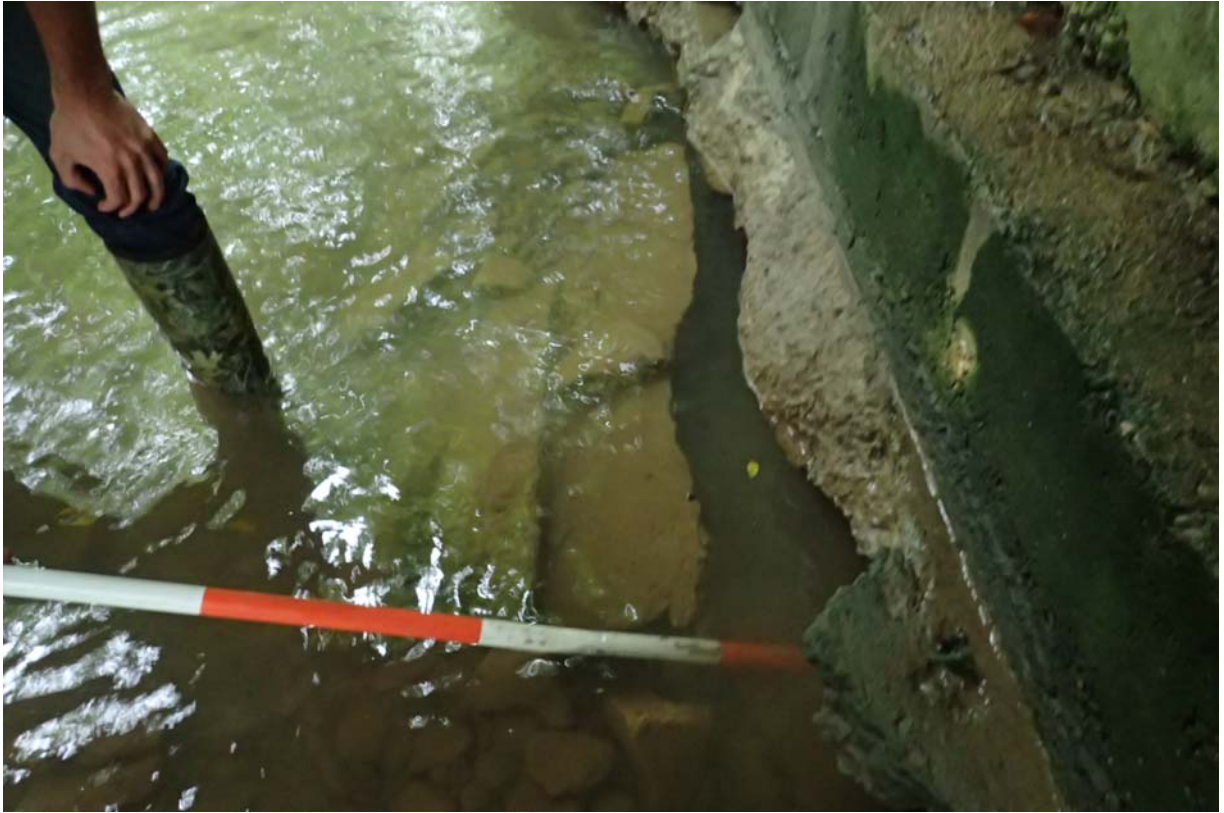
Approximate 1' of horizontal undermining of the west abutments footing near midlength.
