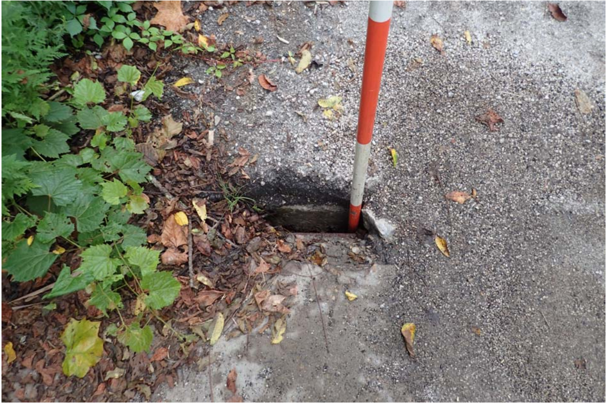
1' x 1' void at the upstream west end of the deck.
