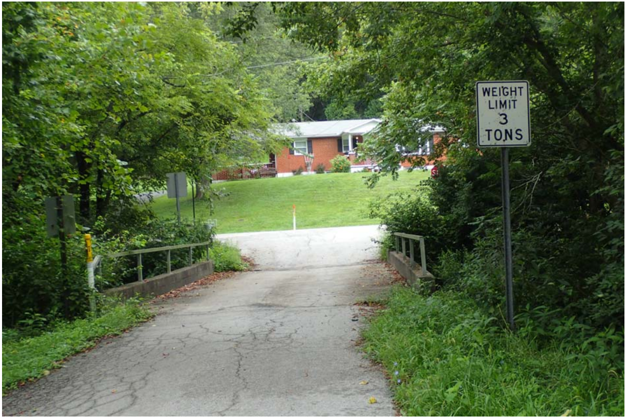
East 3 tons posting.
