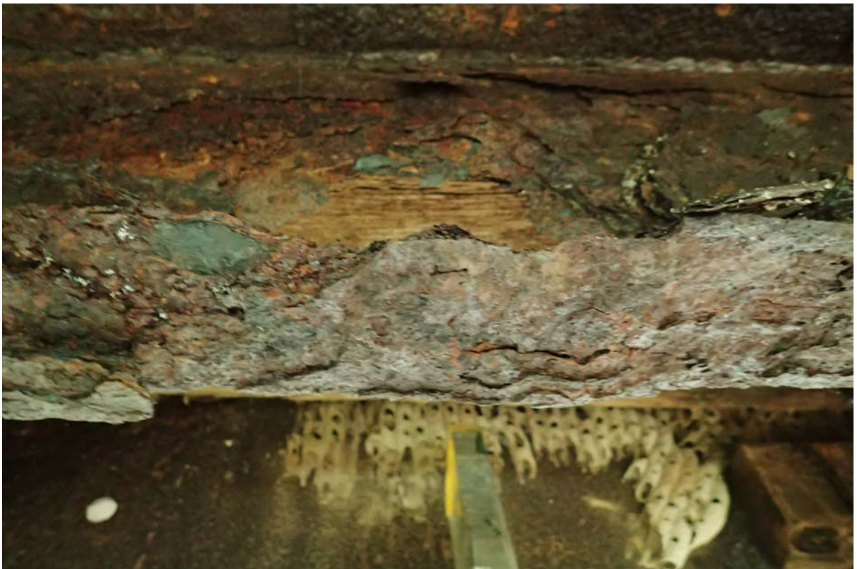
Heavy section loss within the width and thickness of beam 4s bottom flange ~ 7' from the west abutment.
