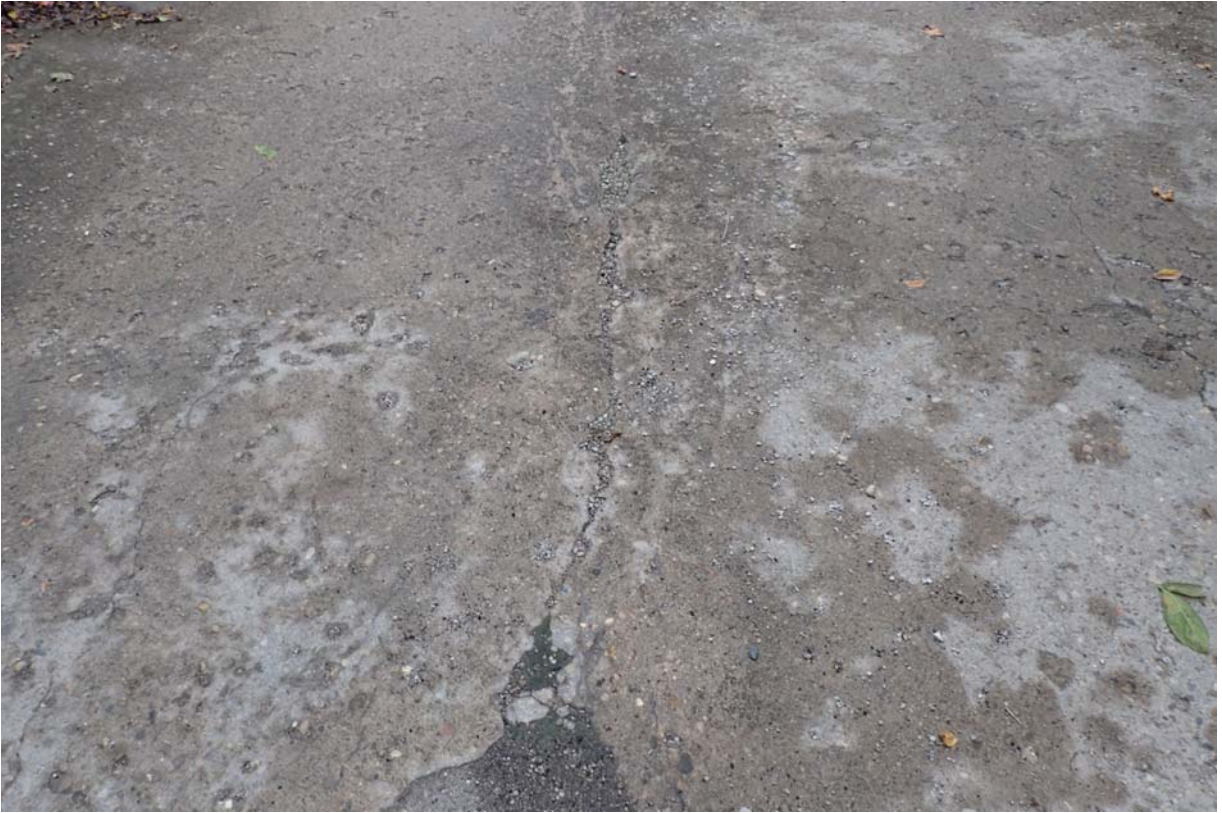
Moderate longitudinal cracking at the east end of the deck along the centerline.
