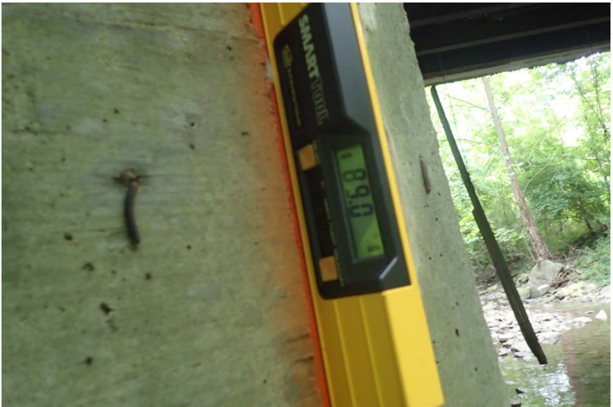
Smart level measurement on the upstream west wingwall.
