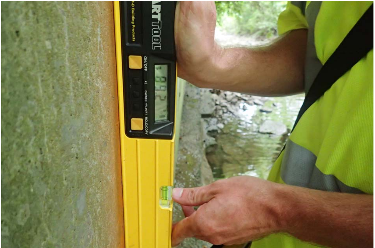
Smart level measurement at the upstream end of the west abutment.
