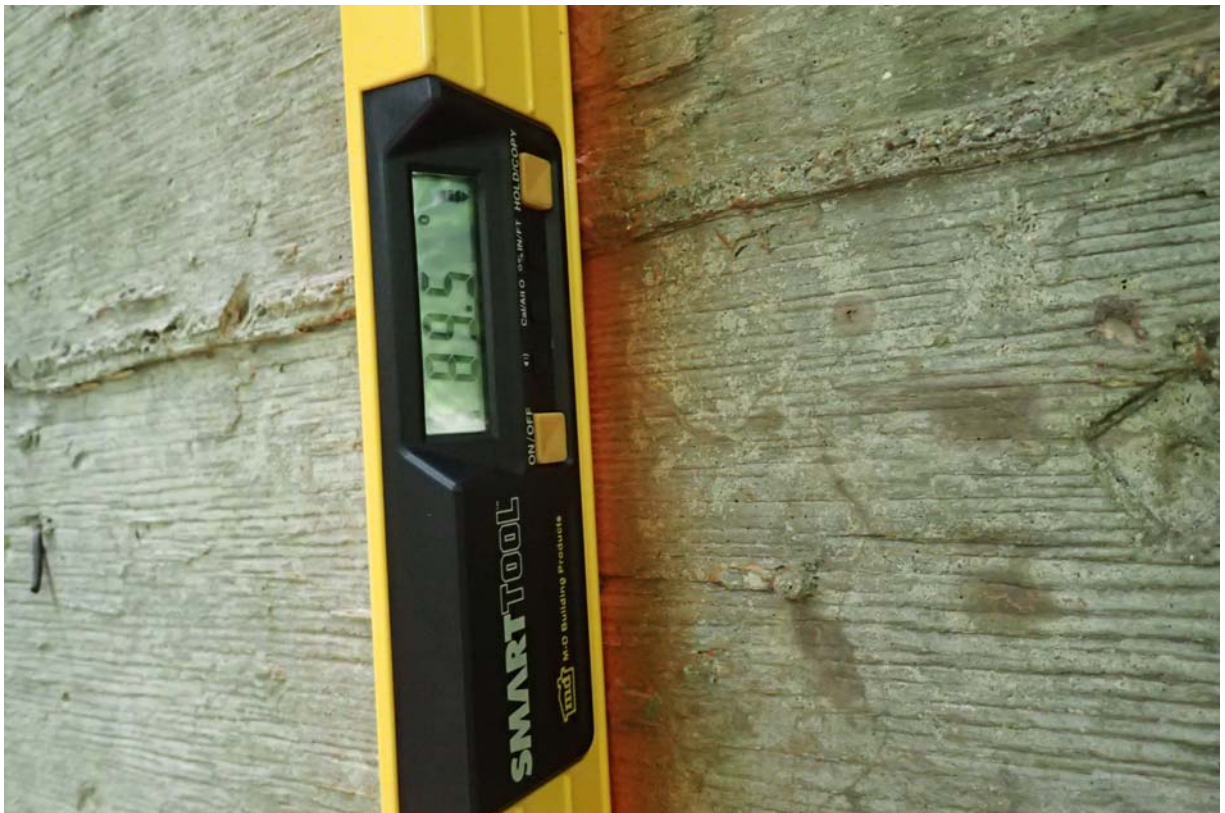
Smart level measurement at the downstream end of the west abutment.
