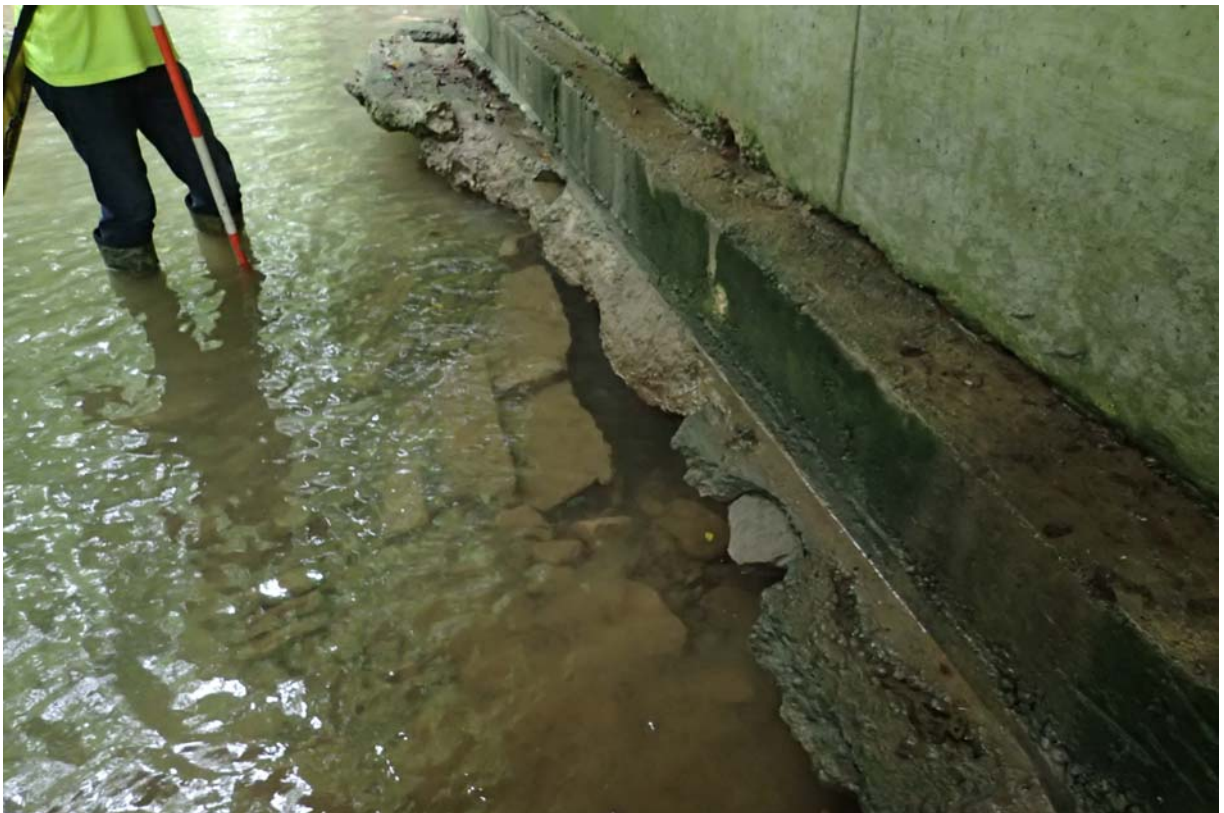
View of spalling and sections broken off of the west abutments concrete protection apron.
