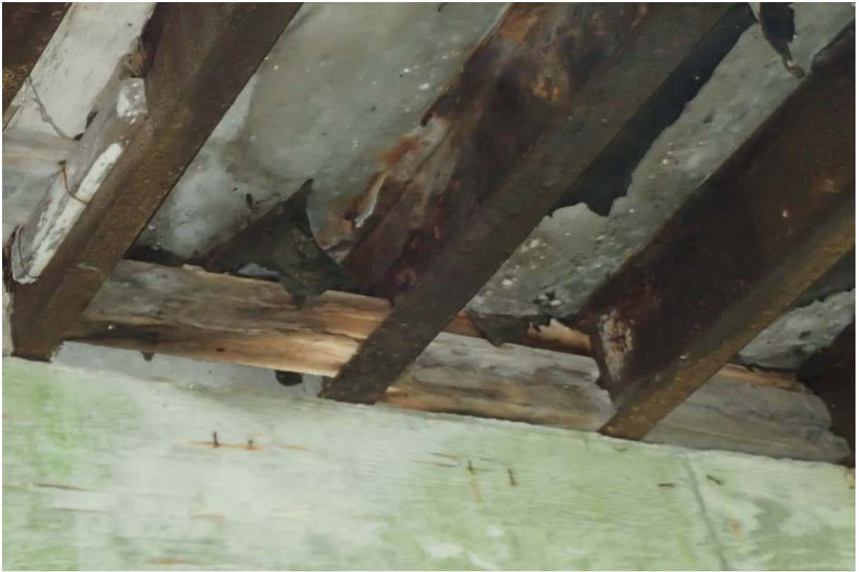
Heavy corrosion at the west end of beam 6 from upstream.
