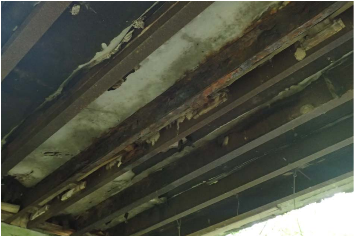
Heavy corrosion along beam 4 from upstream.
