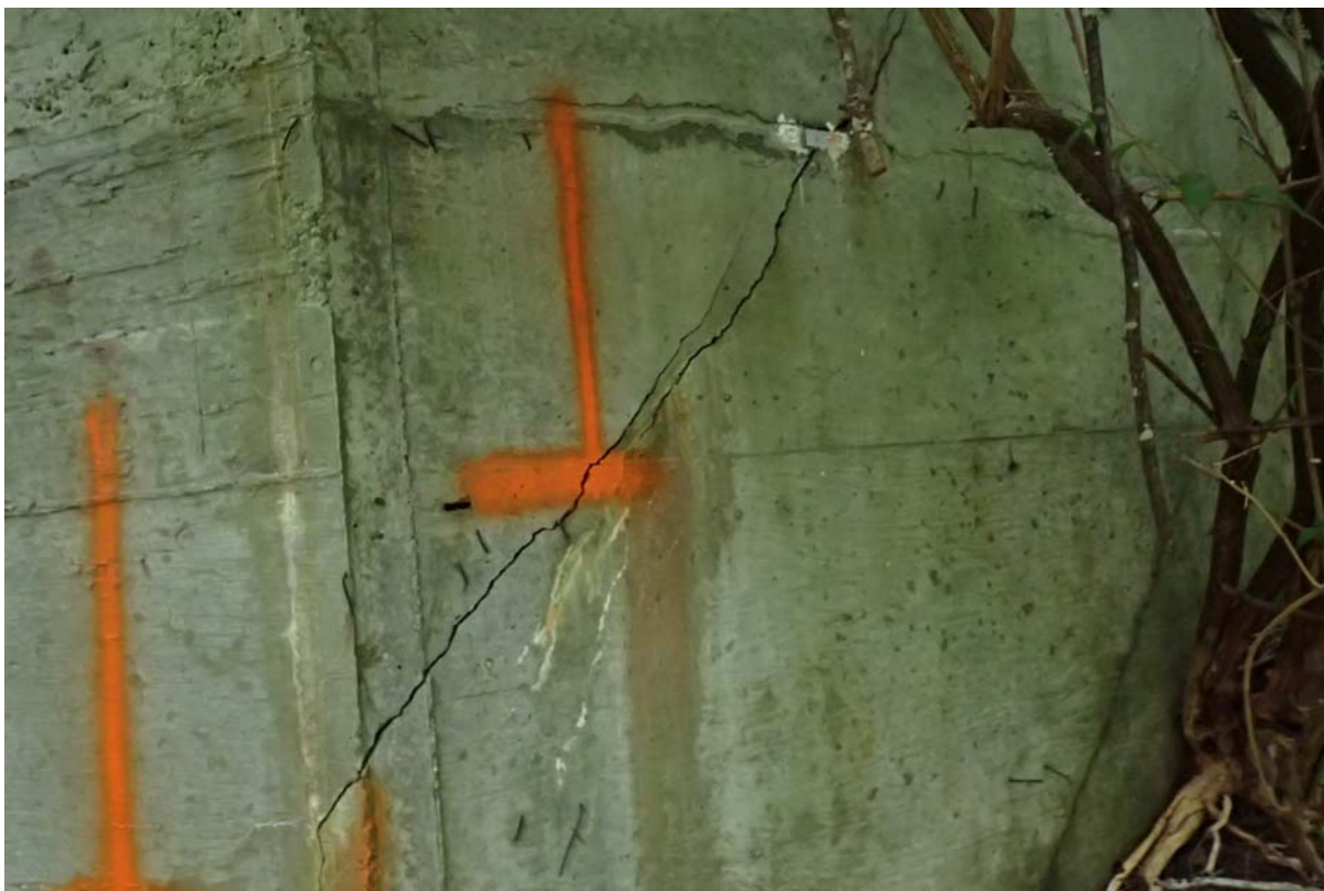
Moderate diagonal cracking ( \sim 3/16'' - 1/4'' ) in the downstream west wingwall.
