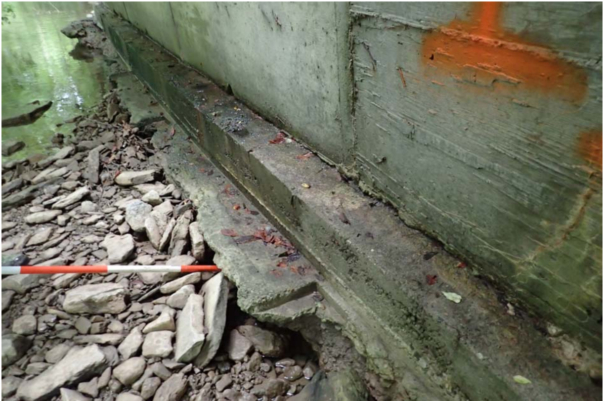
Approximate 6" of horizontal undermining at the downstream end of the west abutments footing.
