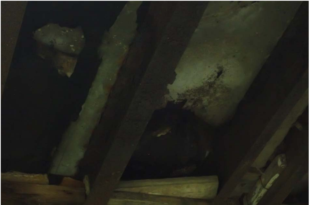
Moderate to heavy corrosion at the west end of beam 3 from upstream.
