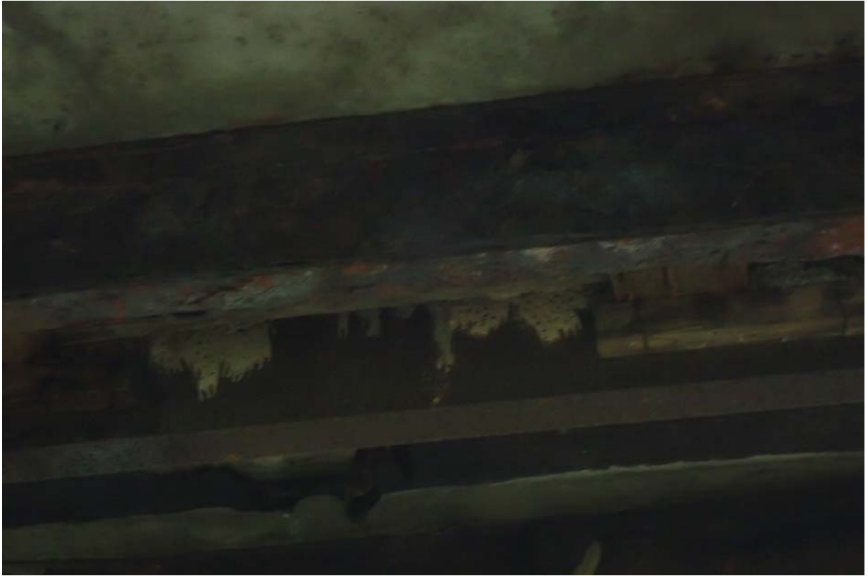
Heavy corrosion along beam 4 from upstream.
