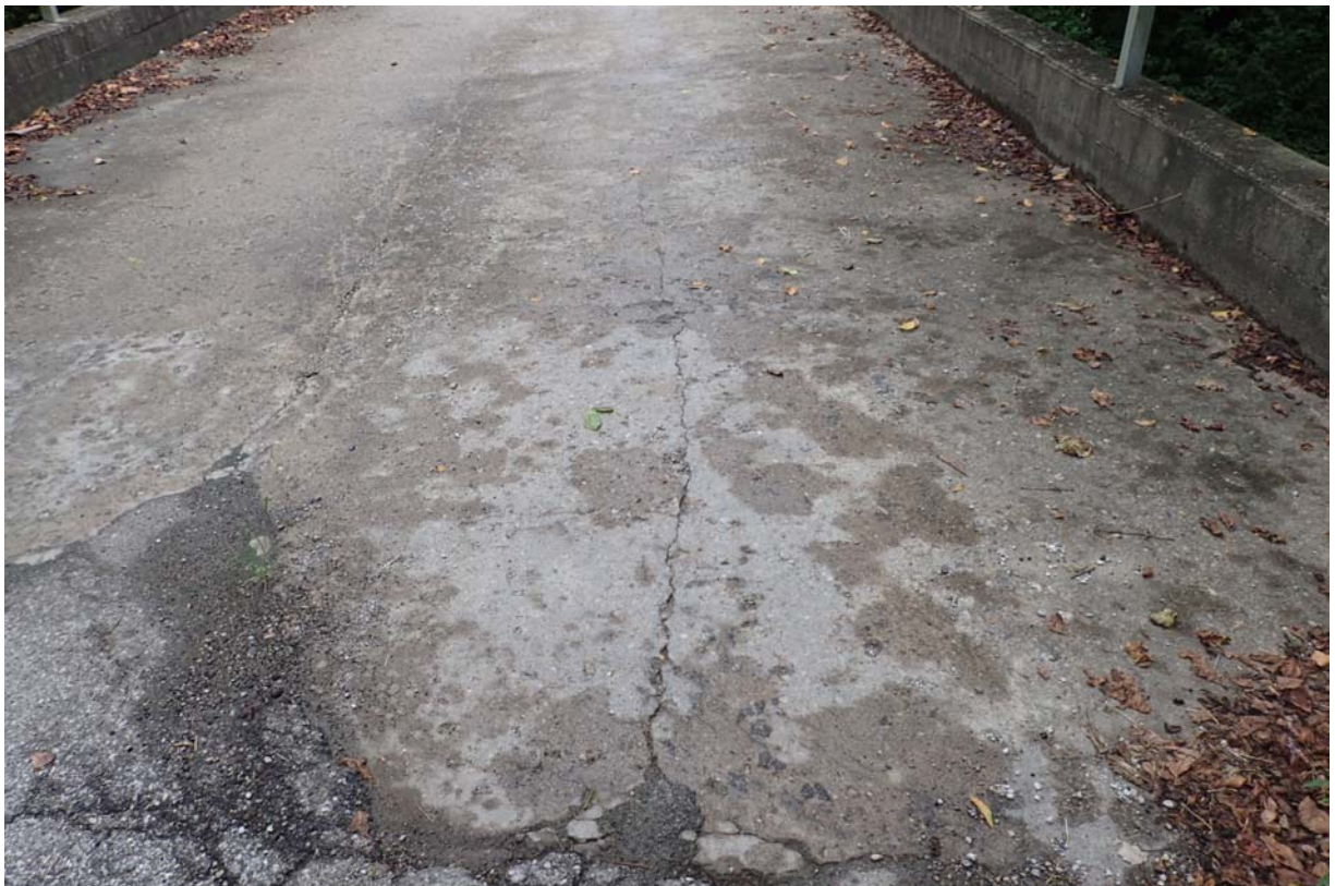
Moderate longitudinal cracking at the east end of the deck.
