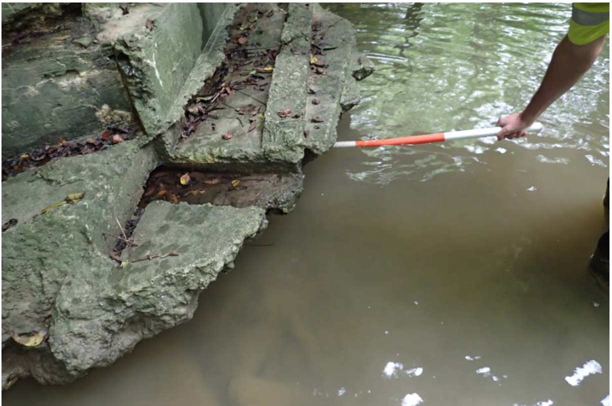
Up to 24" of horizontal undermining at the upstream end of the west abutments footing/apron.
