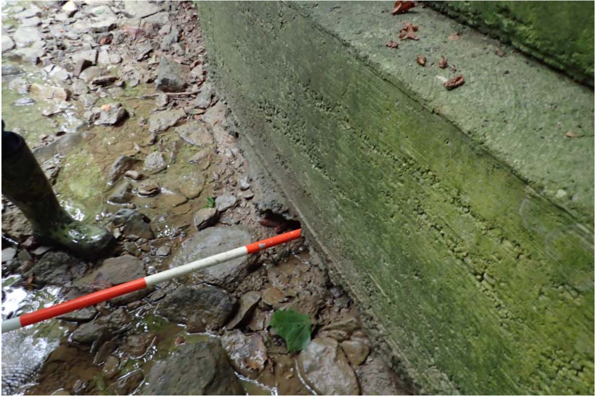
Minor undermining (horizontally up to 5") along the downstream 1/2 of the east abutments footing.
